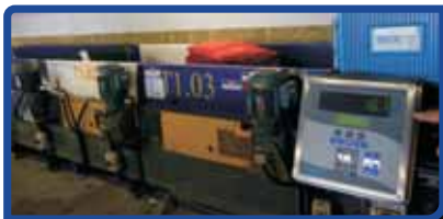
Inline baggage weighing system
